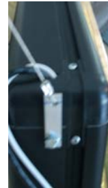
Side view with hanging cables
